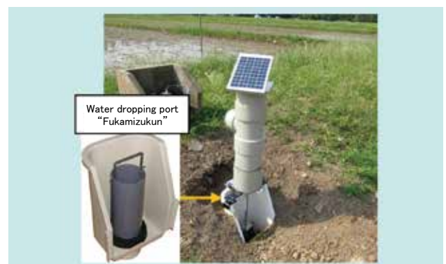
Fig. 7 Installation Example on Drain Side (Fukamizukun)
