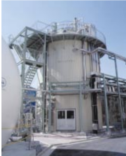
Anaerobic digestion tank in sludge recycling plant
