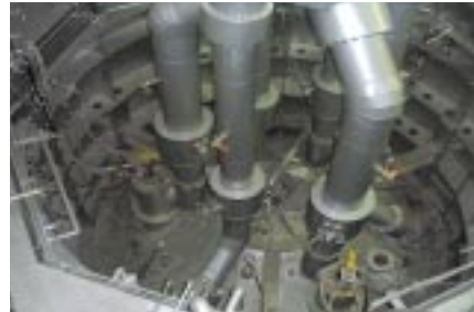
Rotating-type surface melting furnace
