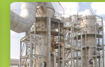
Desulfurization equipment and denitrification
