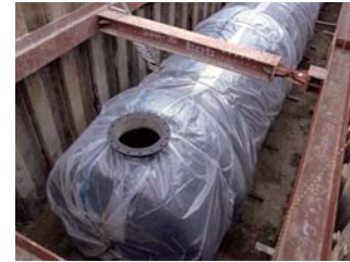
10 Earthquake resistant reservoirs: used to ensure the supply of drinking water when water services are halted due to an earthquake or other disaster.
