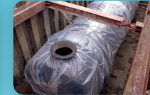
Seismically reinforced water tanks
