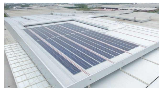
Solar power generation system on the roof equivalent to output 510.3 kW
