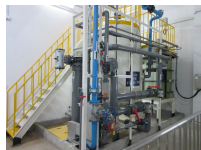
At Kubota Agricultural Machinery (Suzhou) Co., Ltd. (China), we installed recycling treatment equipment for reusing wastewater from processes throughout the entire plant, and this has realized zero emissions of process wastewater.
