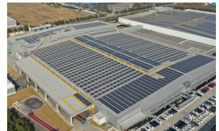
Solar power generation system installed on the rooftop of a plant in China
