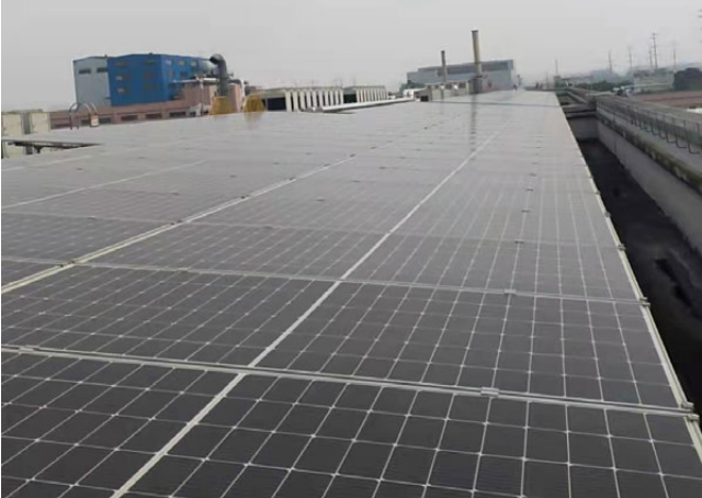
Kubota Engine (WUXI) Co., Ltd. (China) installed solar panels capable of generating 600 kW at its plant premises. Power generation commenced in September 2021 and the amount generated annually will correspond to 20% of all electricity used.
