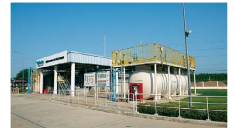
This state-of-the-art KET plant features an effluent-free system to reduce environmental load.
