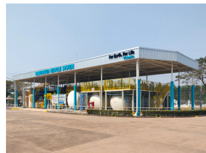
Kubota Engine (Thailand) Co., Ltd. has added additional capacity to its wastewater treatment system with the use of a membrane bioreactor (MBR). Recycled water is being used to water the gardens around the plant and as domestic water.
