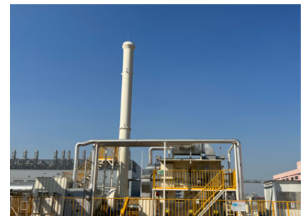
Kubota Engine (WUXI) Co., Ltd. (China) has installed a regenerative thermal oxidizer (RTO) and is working to reduce its VOC emissions.
