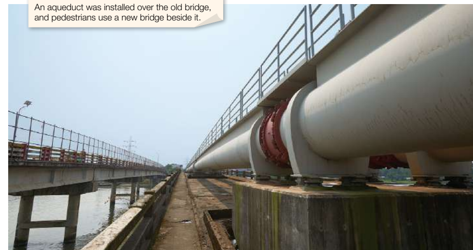
An aqueduct was installed over the old bridge, and pedestrians use a new bridge beside it.
