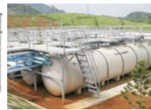
● Wastewater treatment plant (Johkasou)
