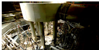
Rotary-type surface melting furnace that can liquefy residue and ash, turn it into a slag, and reuse it as a resource
