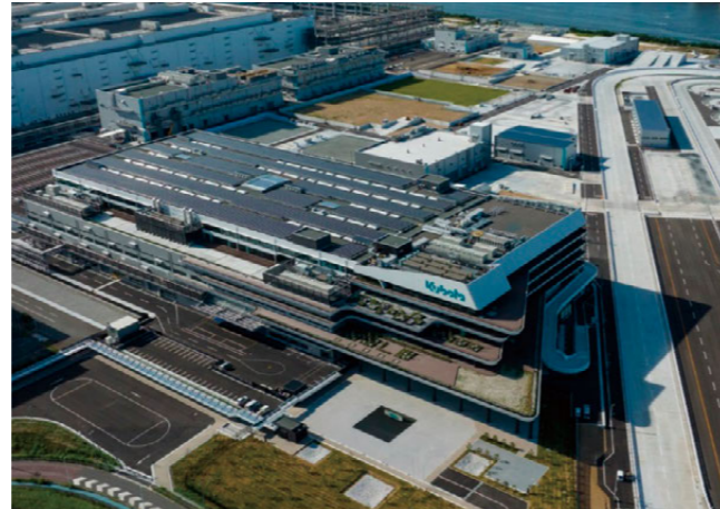
Solar panels capable of generating 1,566 kW of power were installed at the Kubota Global Institute of Technology (Japan), a facility that opened in September 2022.
