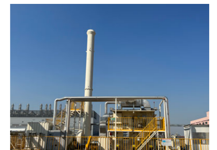
Kubota Engine (WUXI) Co., Ltd. (China) has installed a regenerative thermal oxidizer (RTO) and is working to reduce its VOC emissions.
