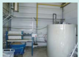
Effluent treatment equipment
