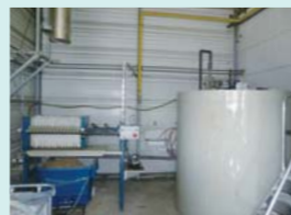
Effluent treatment equipment
