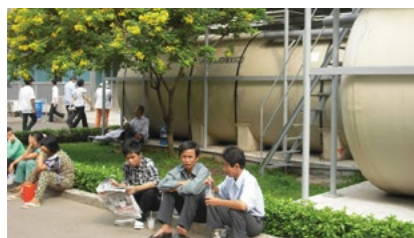
Urbanization creates a growing need for sewer and water treatment facilities (This photograph shows a wastewater treatment plant (Johkasou) used in areas without developed sewers)
