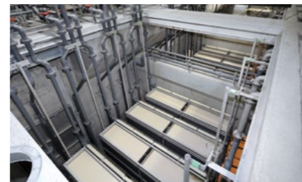
Submerged membranes: used to purify wastewater, including industrial and domestic sewage.
