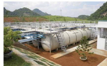
Wastewater treatment plants (Johkasou): used to treat wastewater in areas where there are no sewage lines.
