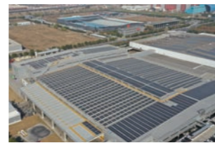
Solar power system installed on the factory rooftop (China)
