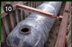
10 Earthquake resistant reservoirs: used to ensure the supply of drinking water when water services are halted due to an earthquake or other disaster.
