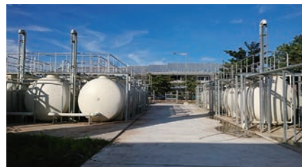
● Johkasou used to treat wastewater in areas where there are no sewage lines.
