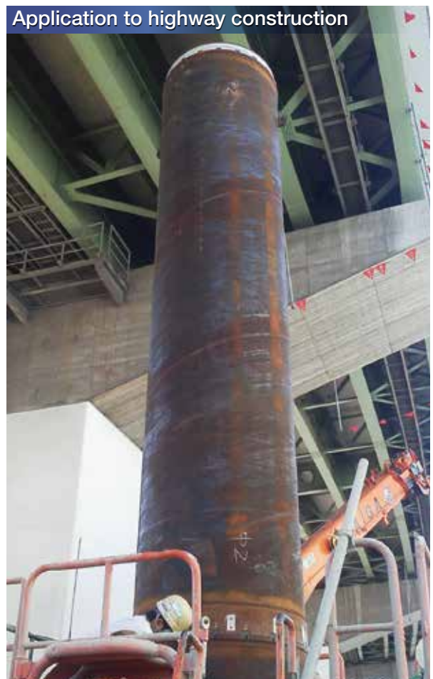
*Example of construction under the condition in which an overhead clearance is restricted.
