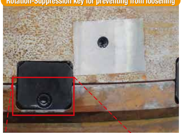
*Number of rotation-suppression keys changes depending on piling methods and construction machinery.
