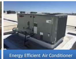
Energy Efficient Air Conditioner
