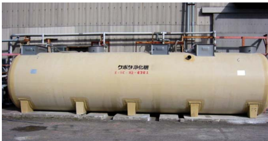
Large-Scale Wastewater Treatment Tank
