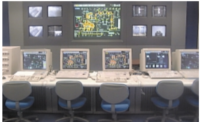
Central control room
