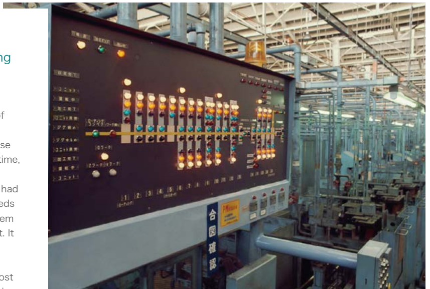
A centralized control monitor installed in the Tsukuba plant
