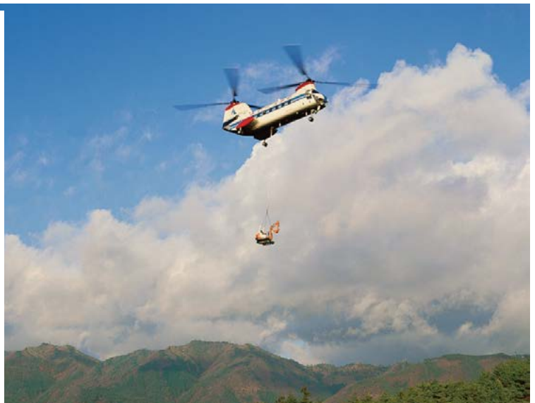
Mini Excavator KH5H being transferred to an electric cable installation site by a helicopter
