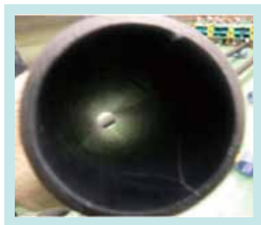
Fig. 5 Inner Surface of Cracked HTPP
