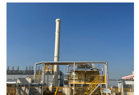
Kubota Engine (WUXI) Co., Ltd. (China) has installed a regenerative thermal oxidizer (RTO) and is working to reduce its VOC emissions.
