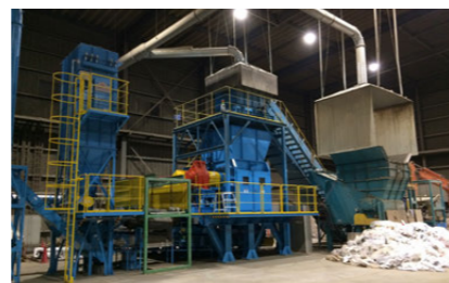
Plastic crushing and sorting facility
