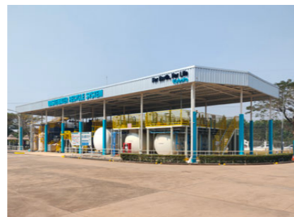
Kubota Engine (Thailand) Co., Ltd. has added additional capacity to its wastewater treatment system with the use of a membrane bioreactor (MBR). Recycled water is being used to water the gardens around the plant and as domestic water.
