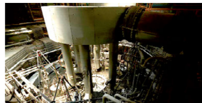
Rotary-type surface melting furnace that can liquefy residue and ash, turn it into a slag, and reuse it as a resource
