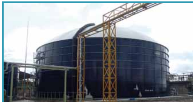
Palm oil mill effluent treatment facilities on order in Malaysia
