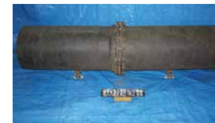
The pipes after 53 years in service
