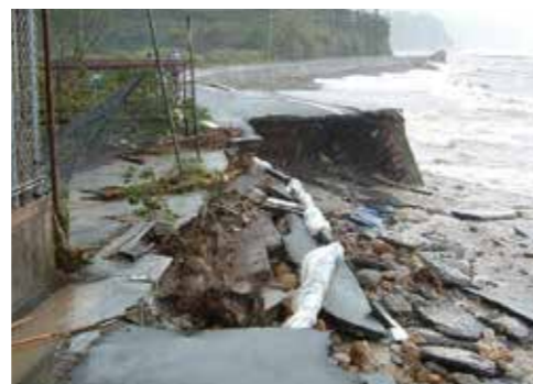
NS-type DN150 (6") after landslide
