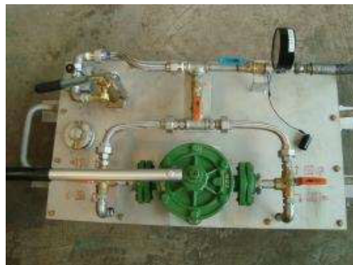
Pict.4 Water Tank and Hand Pump
