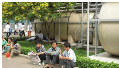
Urbanization creates a growing need for sewer and water treatment facilities (This photograph shows a wastewater treatment plant (Johkasou) used in areas without developed sewers)
