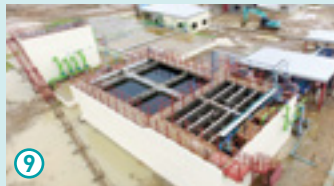
Water purification plant constructed in Thilawa Industrial Park
