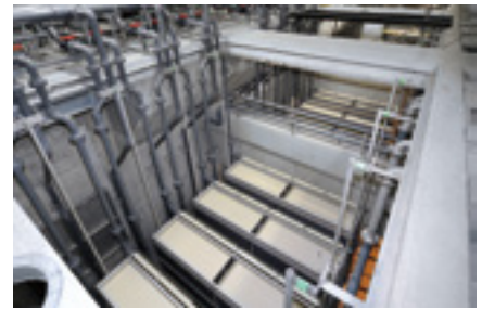
Submerged membranes: used to purify wastewater, including industrial and domestic sewage.
