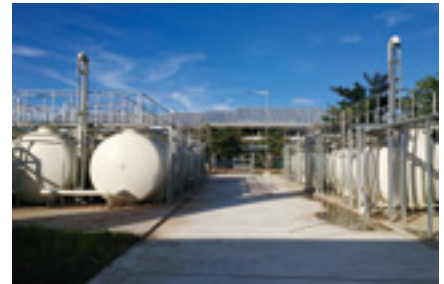
Johkasou: used to treat wastewater in areas where there are no sewage lines.
