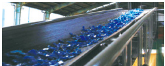
Crushing and recycling plants: used to crush and sort recyclable garbage to enhance its resource value so that it can be reused or turned into raw materials or fuel.
