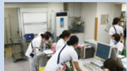
Installed in a nurse station
