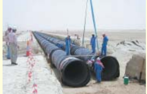
The straight pipes with 1600mm in diameter, 9m in length, the longest in the world, are welded. They are continuing to the horizon.
