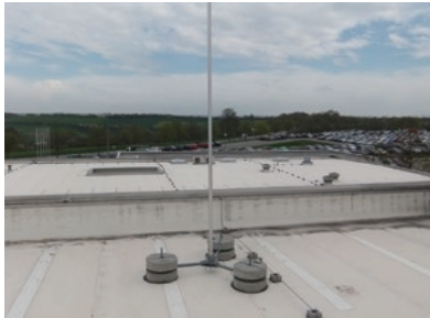
The lightning protection system introduced in response to frequent thunderstorm Kubota Baumaschinen GmbH
